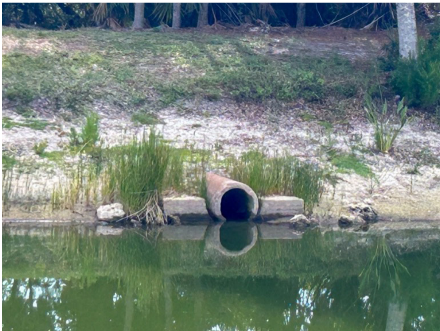
Low water levels on Turtle Pond expose a conduit connection to an adjacent wetland
